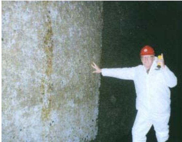
Concrete Wall in Power Plant Cooling Water Intake Coated With GE Exsil™2200 (Uncoated Concrete Wall Surface: Zebra Mussel Build-Up of 4 Inches)
