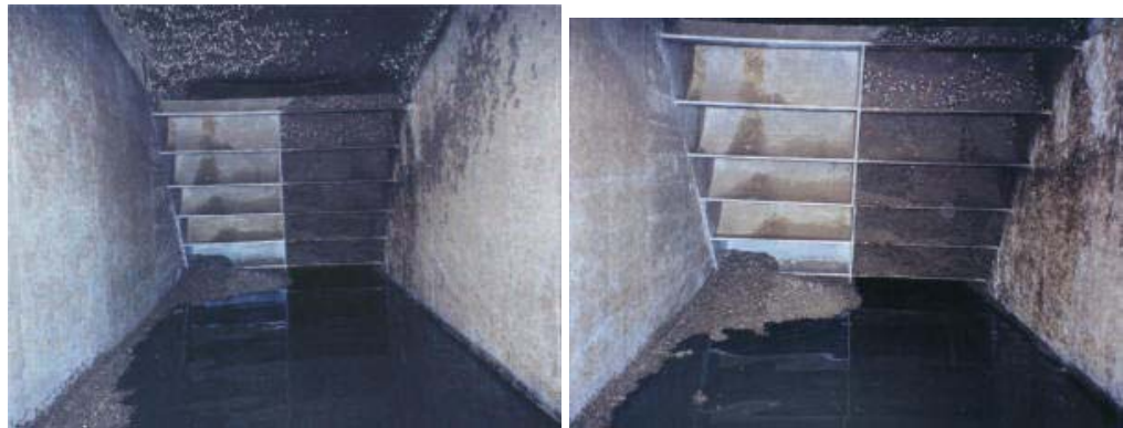
Power Plant Cooling Water Intake- Steel Deflecting Veins (Left Side Coated with GE RTV11: Mussels Came Off When Tunnel Drained; Right Side Uncoated Steel: Covered With Zebra Mussels)
