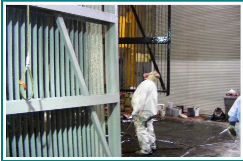
Foreground rack - grayish silicone Tie Coat waiting Top Coat application Background rack - application of black silicone Top Coat in progress
