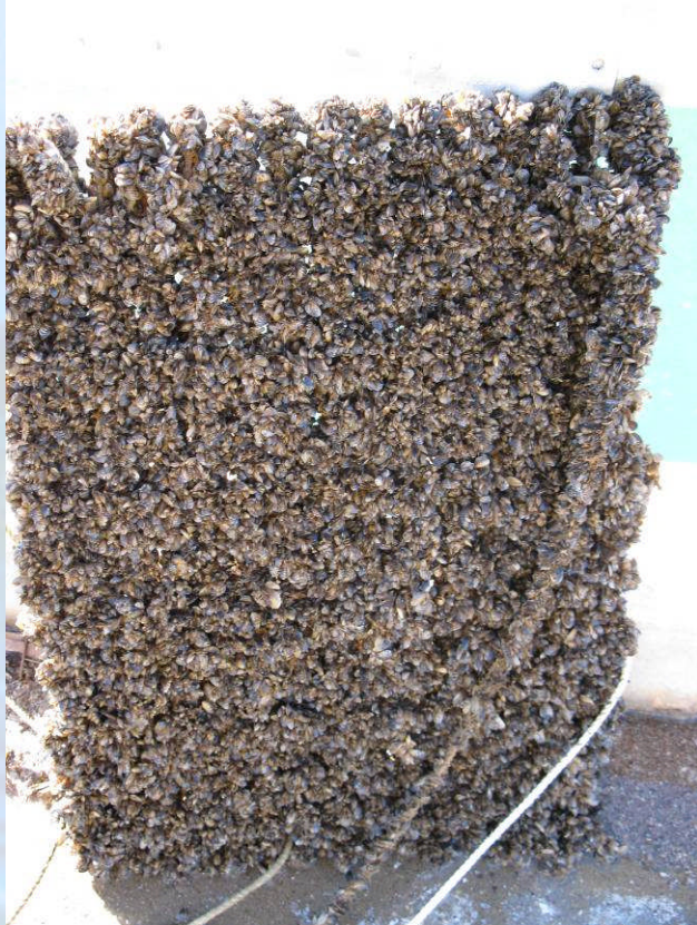
Un-coated Steel Grate – 8/08 through 12/08
